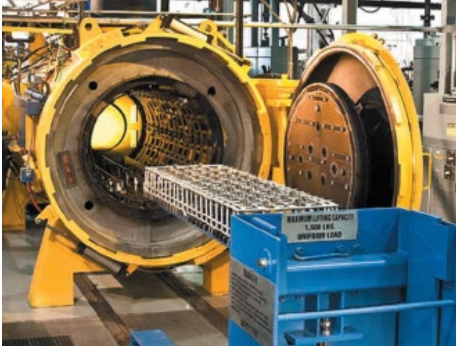
Figure 1: Example of a forming gas metal heat treatment oven
